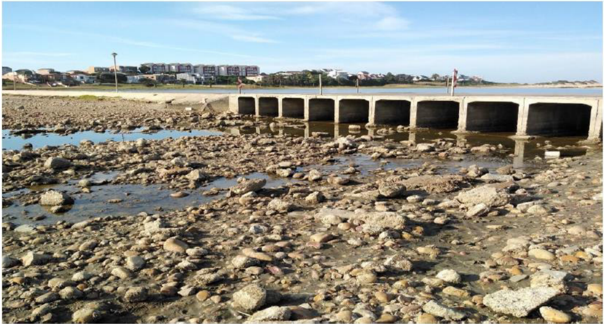
Plate 2. Connectivity between the upper and lower water body was near zero prior to the breach. Picture shows the main causeway across the lagoon. The foreground reflects the large amount of rubble that was deposited in the lagoon over time.
